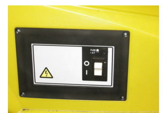
Simple operation on/off switch
